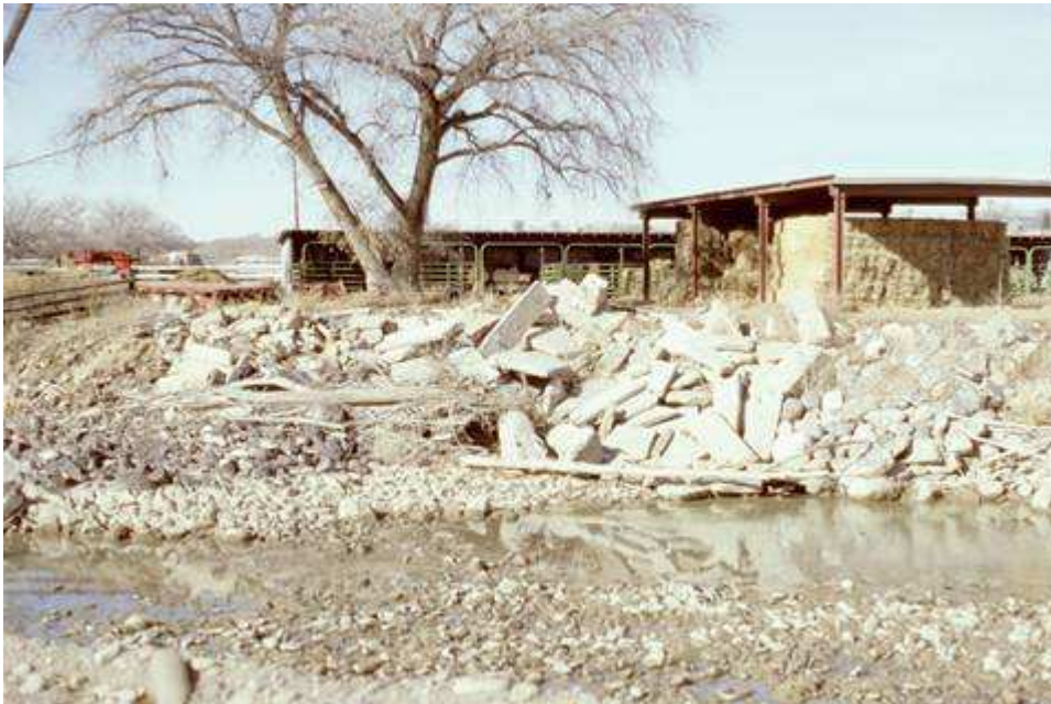
The riverbank adjacent to the property of a private landowner before project construction.
